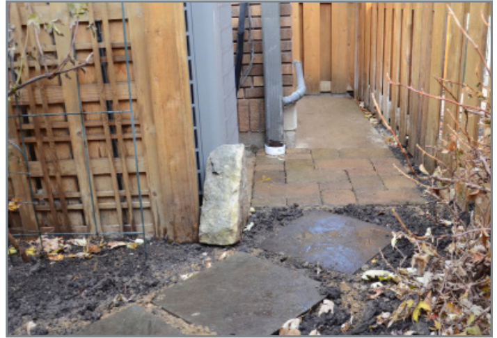
Subsurface infiltration drains, under recently placed pavers, help reduce the amount of rainwater being directed to the private sewer drain, and reduce the risk of water backup in the basement.
